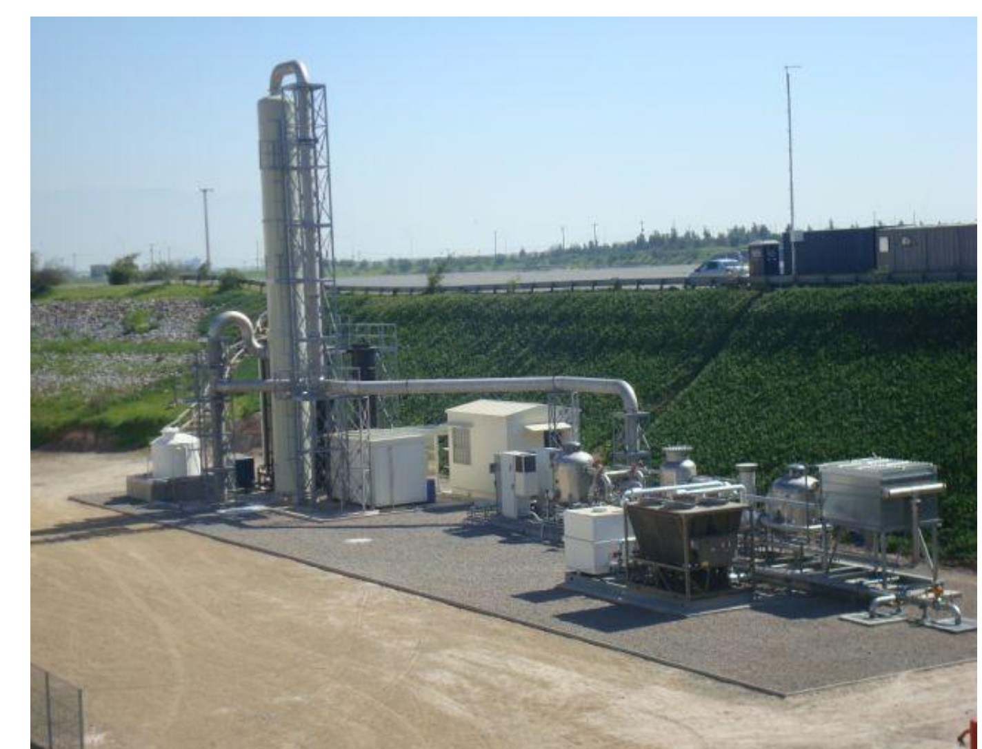
Biogas Treatment Facilities
