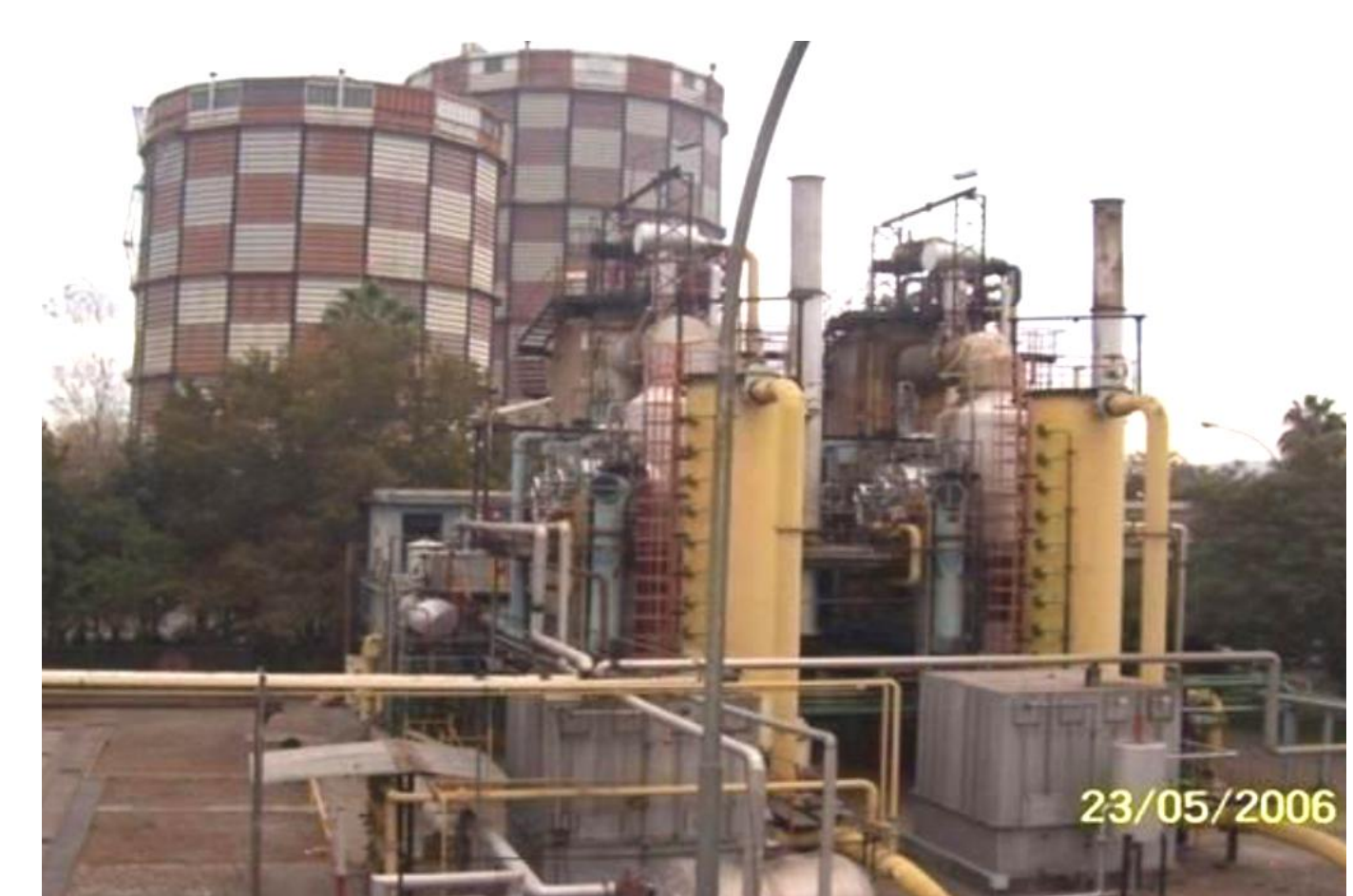
Metrogas Town Gas Plant
