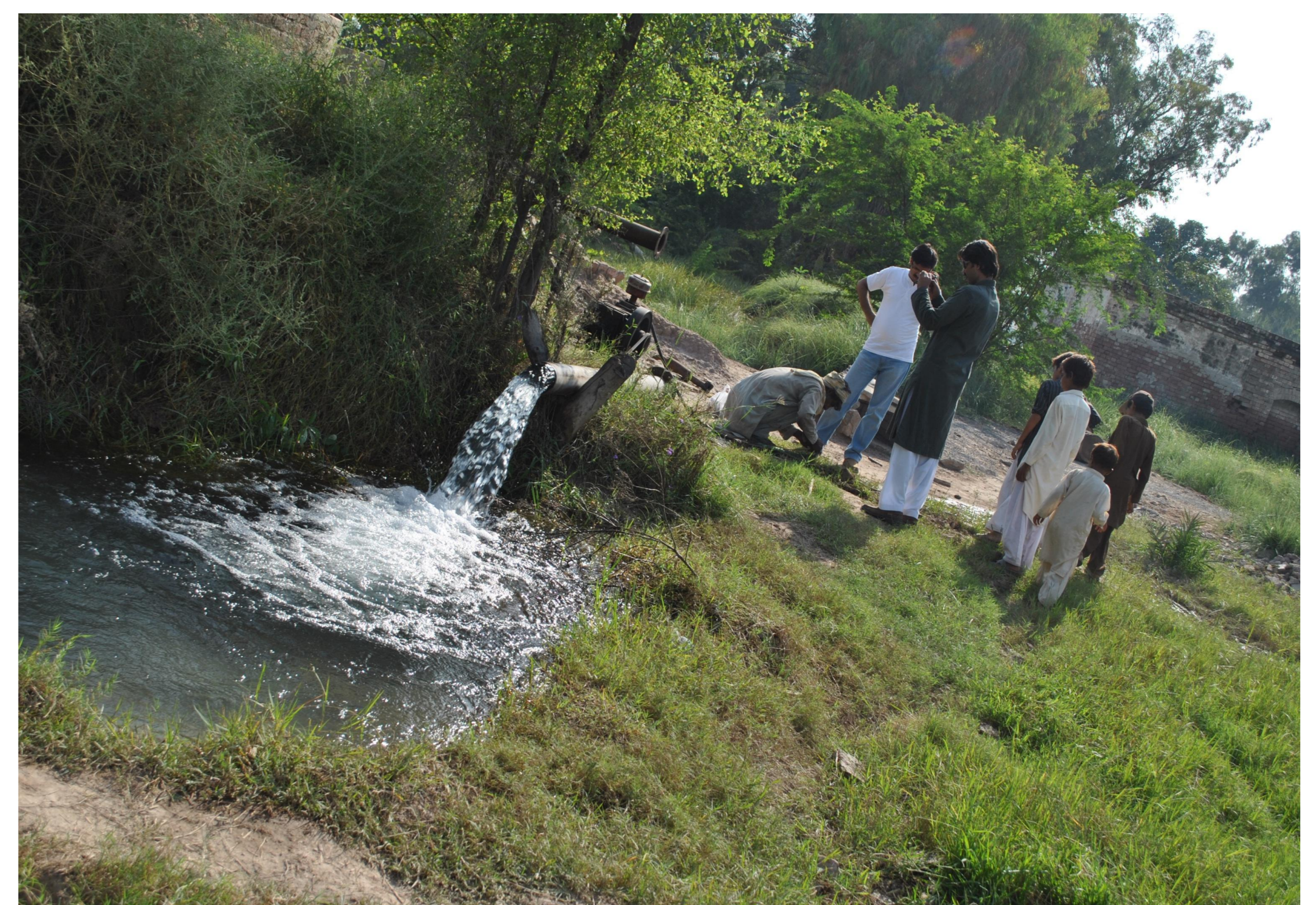
Biogas-Generated Electricity Being used for Water Pumping at KhanKhel Dairy Farm
