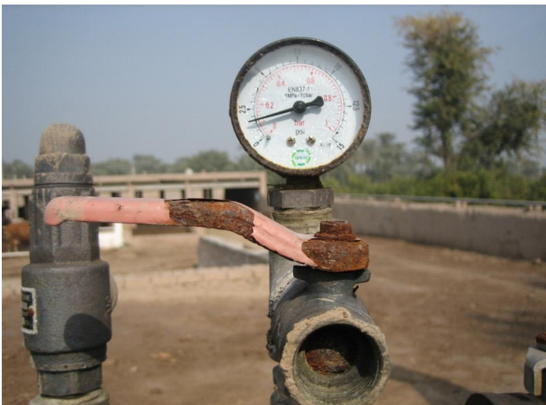
Gas Pressure Valve at 75 m 3 Biogas Plant at Hamidpur Dairy Farm
