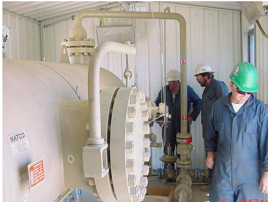
Portable Three Phase Separator, Source: BP
