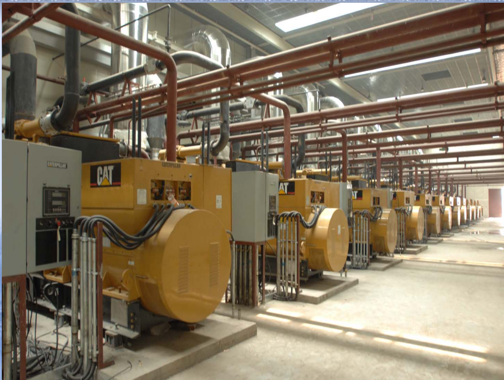
图 晋城120MW煤层气电厂 Fig 120 MW power plant in Jincheng
