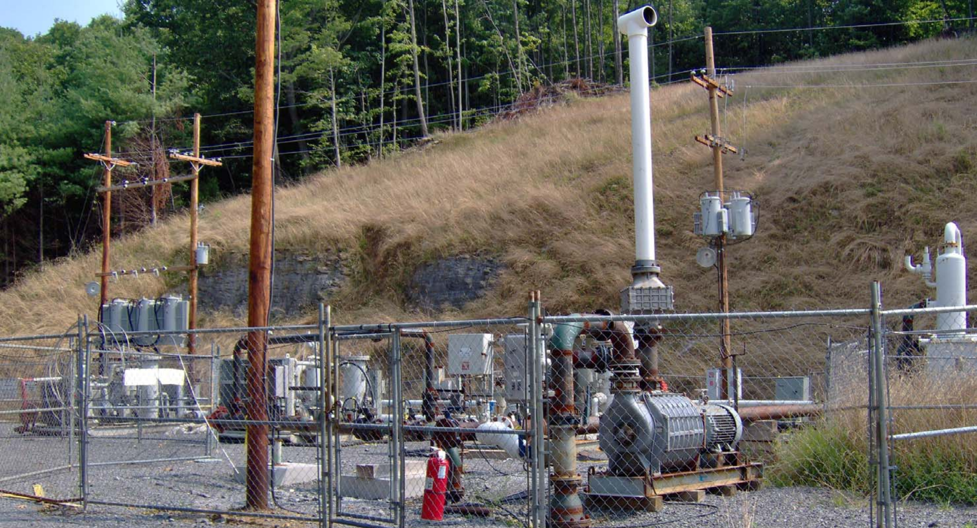
Gob well blowers and compressors
