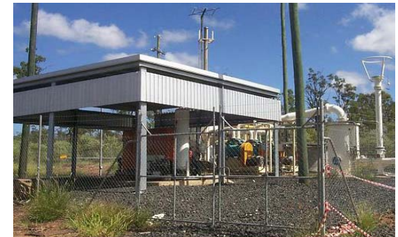
Gas drainage plant
