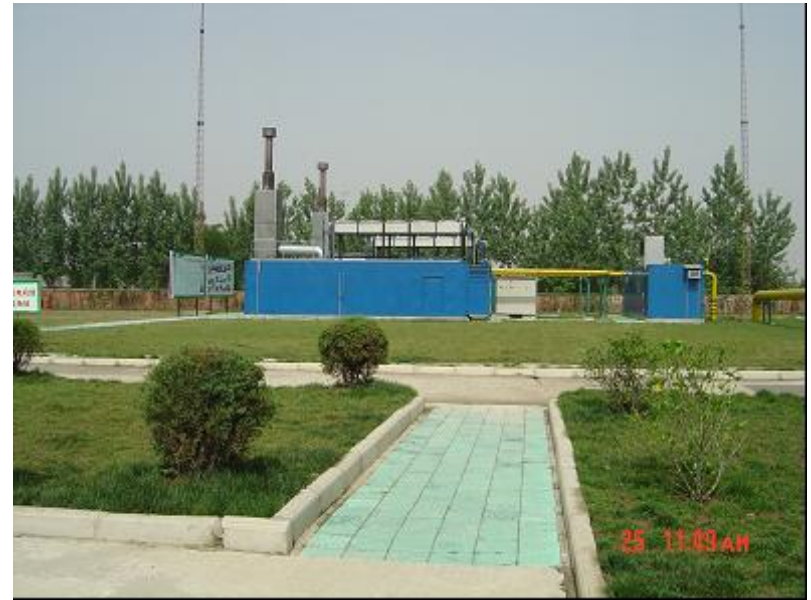
The 2 x 1360 kW gas engine units at the Panyi mine
