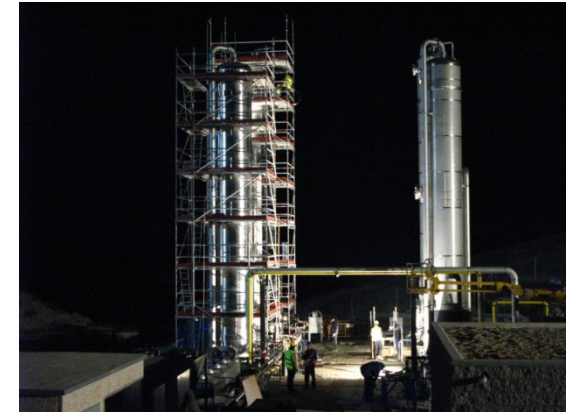
Greenlane® Biogas Upgrading Plant – Madrid, Spain
