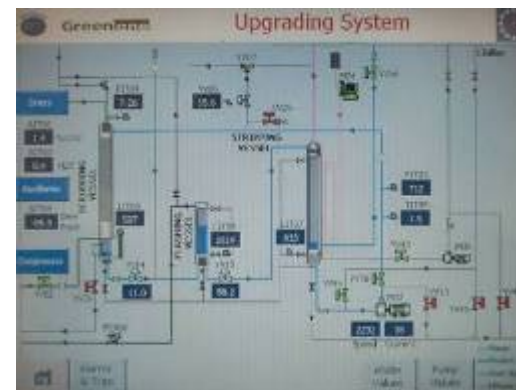
Flotech – AfterCare Remote Monitoring
