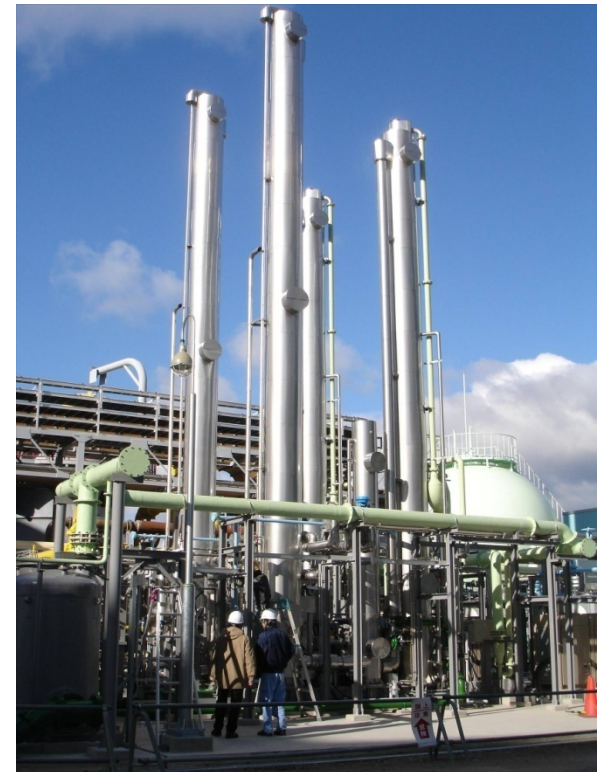
Greenlane® Biogas Upgrading Plant Kobe, Japan (2006)
