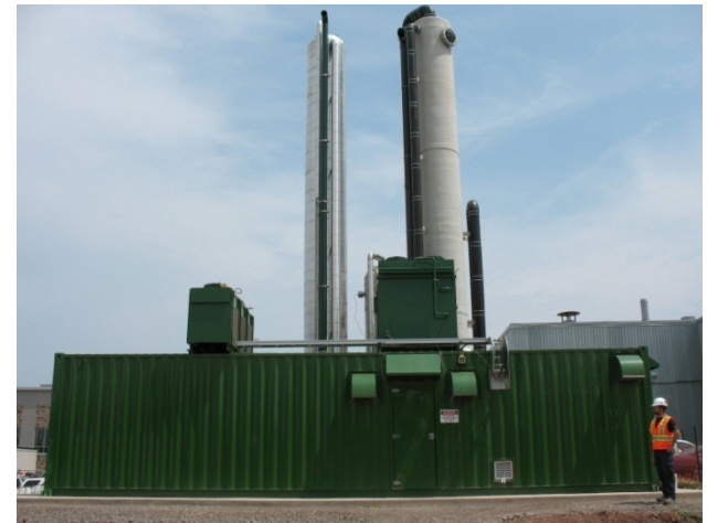
Greenlane® Biogas Upgrading System Hamilton, Ontario
