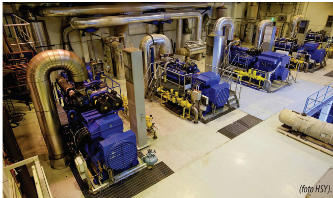
Combined heat and power plant, Viikinkaari WWTP (Helsinki, Finland)
