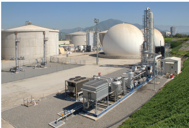
Anaerobic digesters and biogas treatment facilities, La Farfana WWTP (Santiago, Chile)
