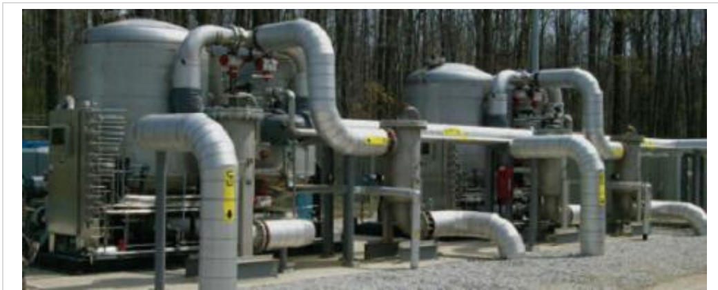
Figure 4-11. Siloxane removal systems at the Lorraine power station at Oberlin, Ohio, USA
