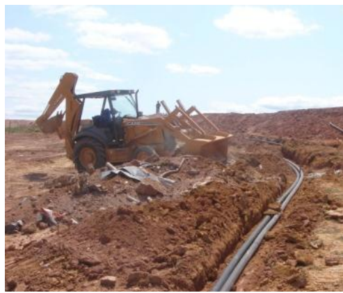
Figure 4-1. Installing a HDPE LFG pipeline for the Brazil MARCA Landfill in Cariacica, Brazil
