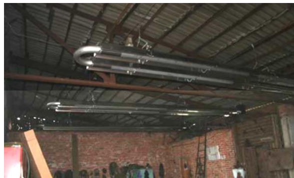
Figure 4-4. Infrared Heater at the Khmelnitsky Landfill in Ukraine
