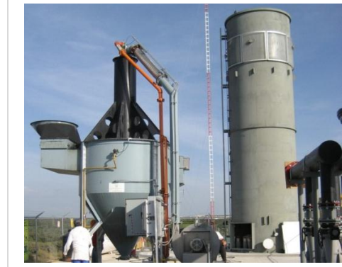
Figure 4-5. Leachate Evaporator System at El Verde Landfill in León, Mexico
