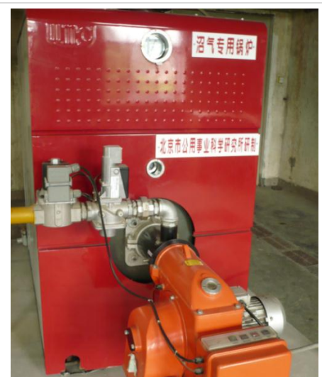
Figure 4-2. LFG Water Boiler System at the Gaoantun Landfill in Beijing, China
