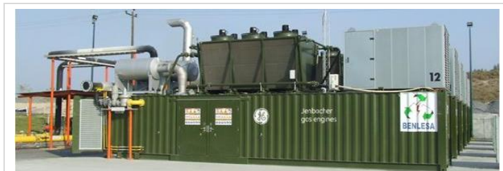
Figure 4-6. GE Jenbacher Internal Combustion Engine at Simprodeso Landfill in Monterrey, Mexico
