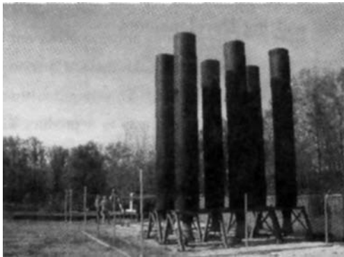
Exhibit 4. Main North Shaft Flares
