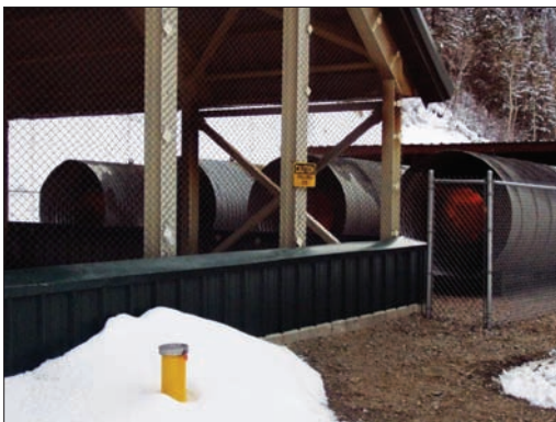
Medium to High Concentration Methane Used for Intake Ventilation Air Heating
