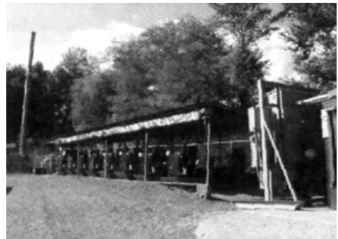
Exhibit 2. Gensets at Nelms Mine
