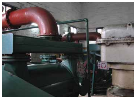
Pumping station at a coal mine under study in China.
