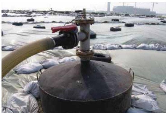
A landfill gas well in China.
