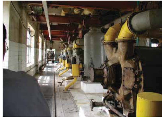
Degasification pumping station at a Ukrainian coal mine.
