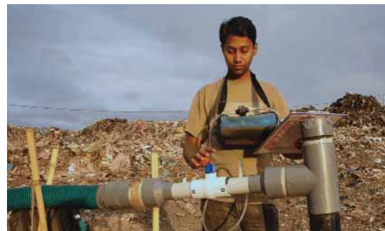
Extraction well monitoring at the Uruli Devachi Landfill in Pune, India.
