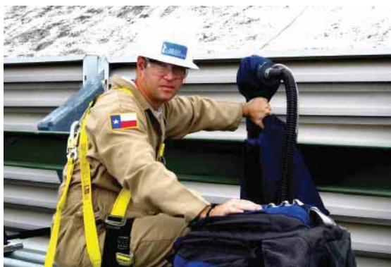
A PEMEX engineer takes a measurement of newly installed dry gas seals at facility in Mexico City, Mexico.
