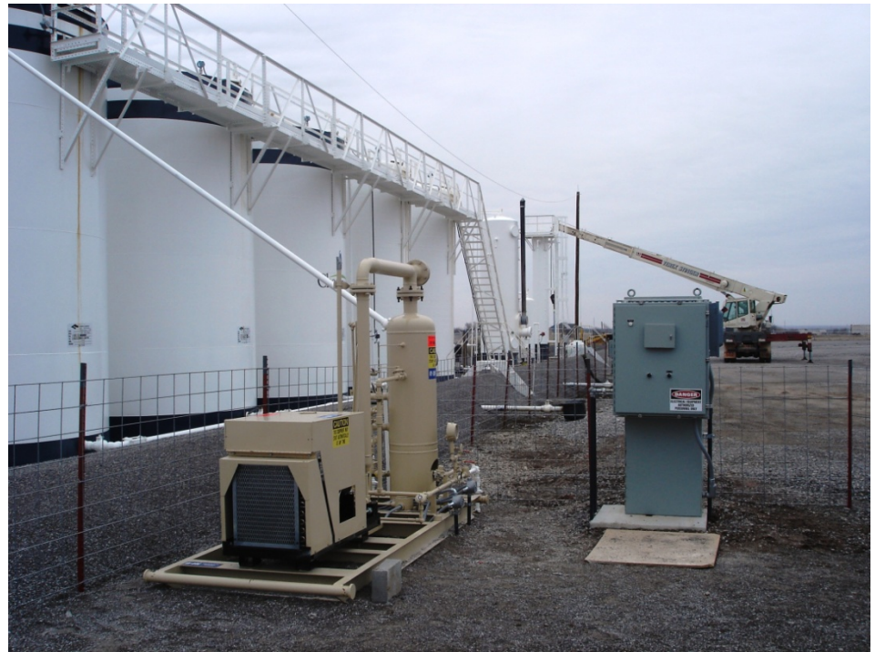
Scroll VRU Installation
