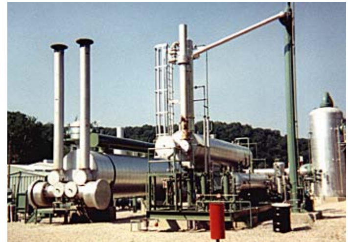
Glycol Dehydrator Unit Source: GasTech
