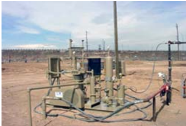
Vapor Recovery Unit – To reduce/eliminate tank flash emissions
