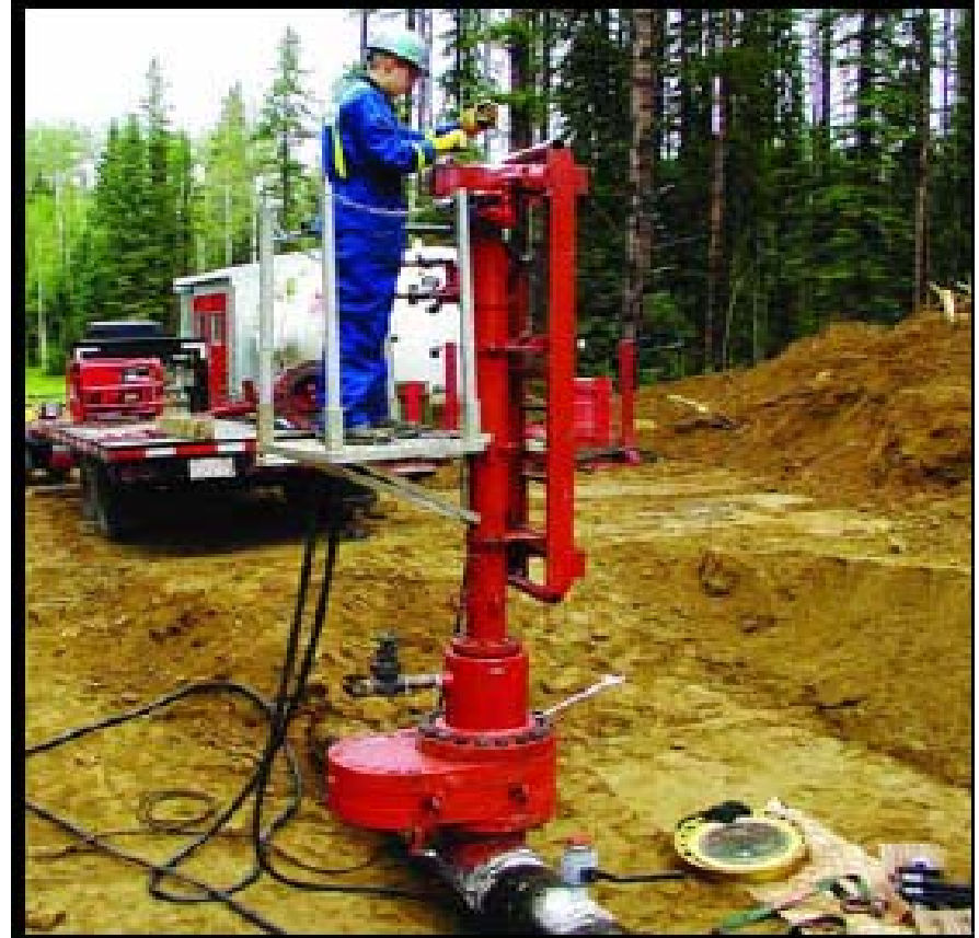
Certified Williamson Industries Technician performing a hot tap with a 760 Tapping Machine as part of a 12" Stopple application.
