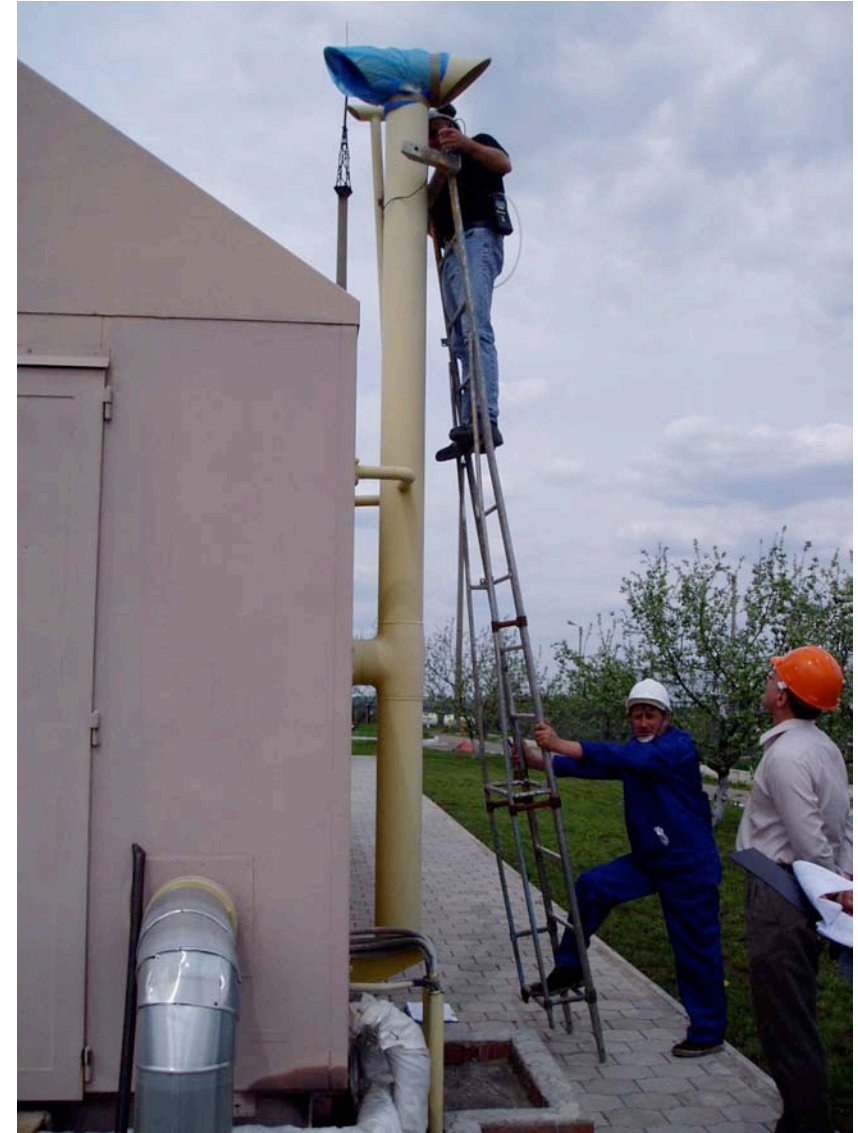
Measurements at Vent Stacks
