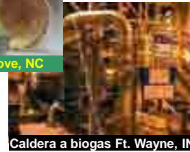
Caldera a biogas Ft. Wayne, IN
