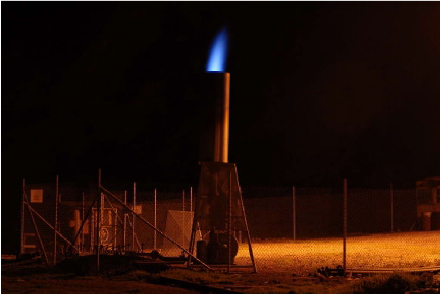
An active flaring methane system at the Zambiza LFG Project Quito, Ecuador
