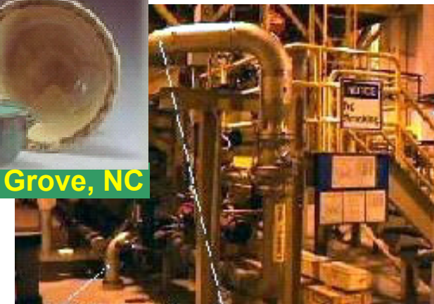
LFG-fired Boiler Ft. Wayne, IN
