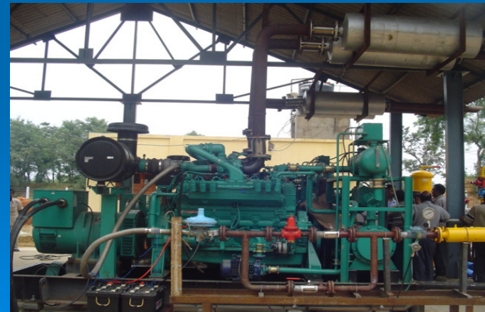
Gas Based Generator at Moonidih
