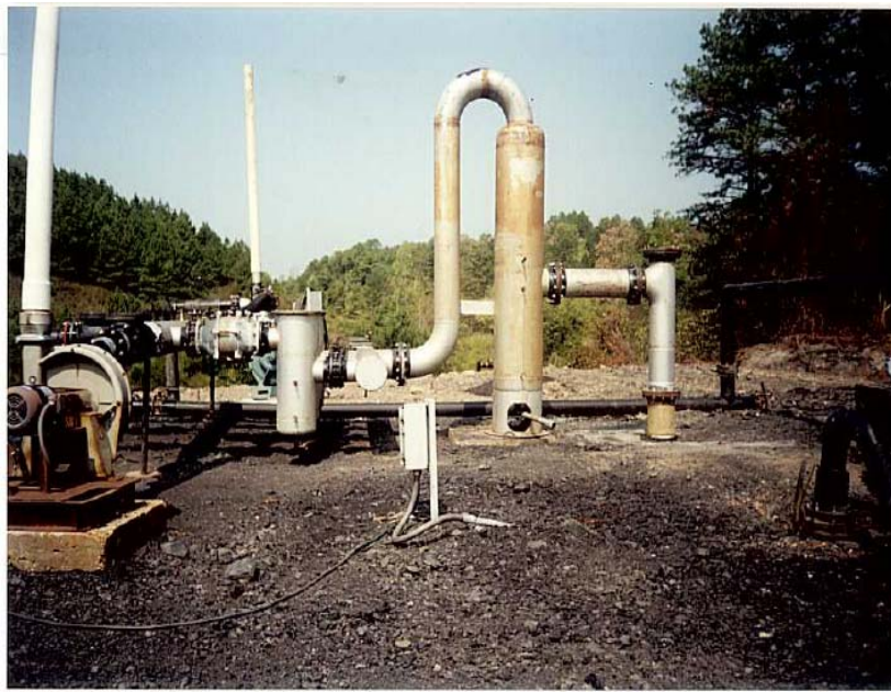
Gob gas plant
