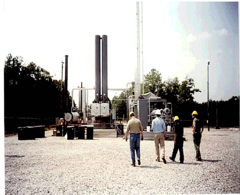
Gas compression Station
