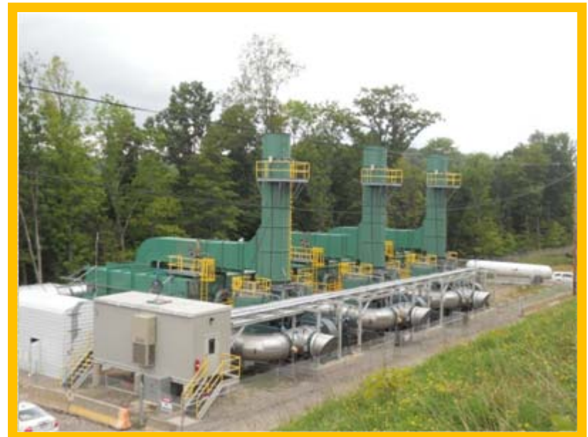
Dürr EcoVAM® McElroy Mine West Virginia
