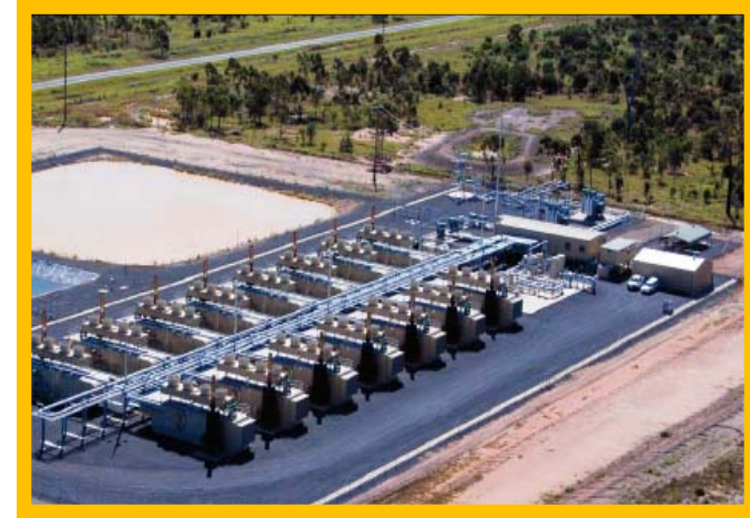
Moranbah North Power Station
