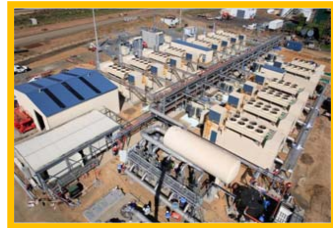
German Creek Power Station
