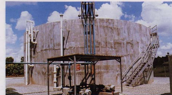
Anaerobic Sludge Digester
