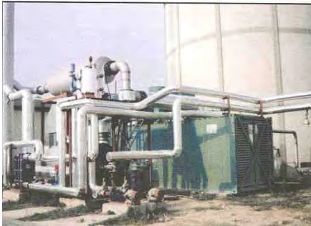
Gas engine with associated piping network
