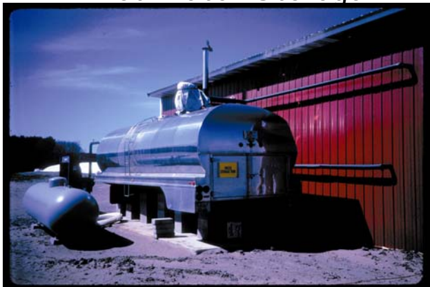
Hot Water Storage
