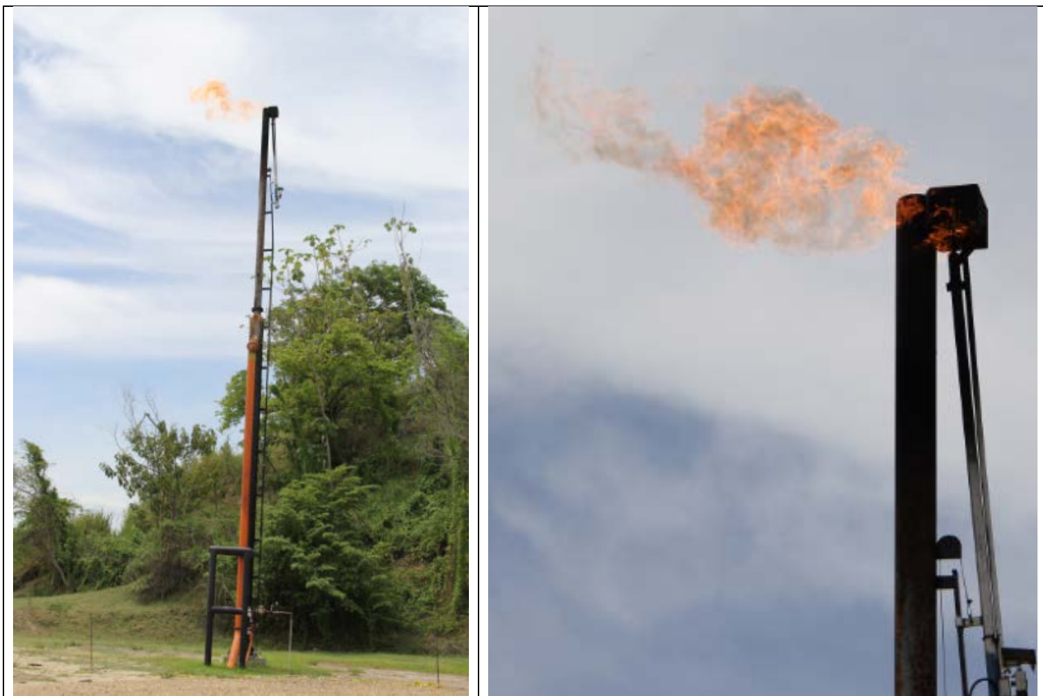
Figure 1: Photographs, of the treater off-gas flare at the CCAC.1 thermal heavy oil central treating facility, 16 August 2015.
