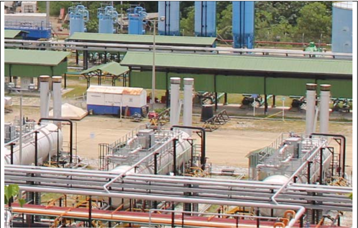
Figure 2: Photograph showing signs of soot accumulation on the two right-most flue stacks at the CCAC.1 central treating facility.
