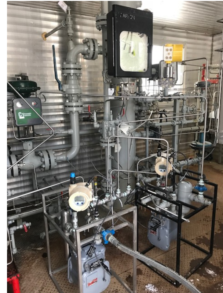
Can it be used in a building where its Div1/Zone1(0) ?
