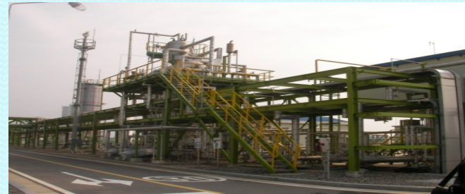
Coal chemical plant-SNG
