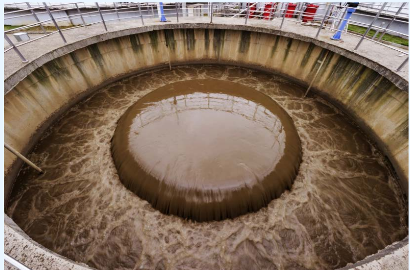
Modern urban wastewater treatment plant Source: hxdyl on Shutterstock (#166378049)
